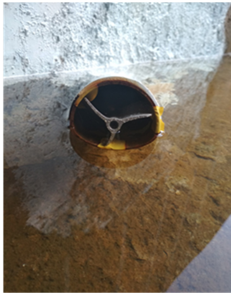
Fig. 3. Single-port submerged diffuser obstructed by fixed vanes.
